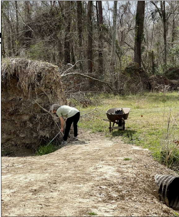
Sue Broussard works on the culvert that she helped to get installed
